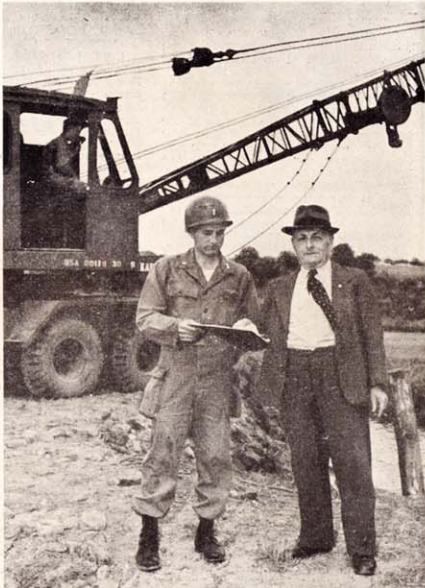
BRIDGE BUILDING AMBASSADORS of the 4th Engr Bn constructed a bridge for use by residents of Windecken as one of several similar completed during the year. 2d Lt Charles L. Stedham discusses plans for the bridge with Burgomeister Franz Paul. —4th Sig Co Photo
